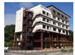
Post-tsunami remains of the Taro Kanko Hotel
